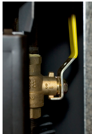
Fig. B15-2 - Gas shutoff valve (typical)
