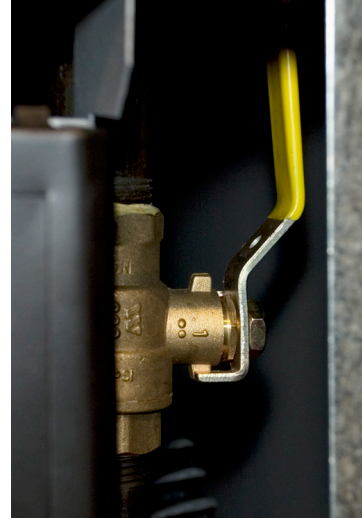
Fig. B23-1 - Gas shutoff valve (typical)
