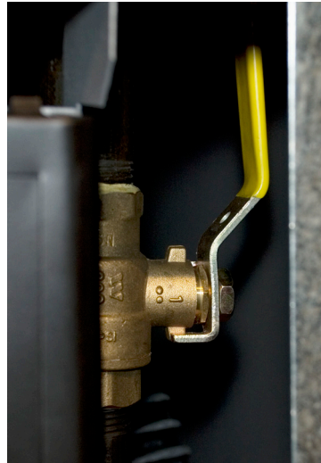
Fig. B11-1 - Gas shutoff valve (typical)
