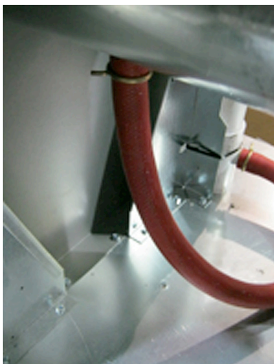
Fig. C5-14 - Drain hose connected under the heat exchanger
