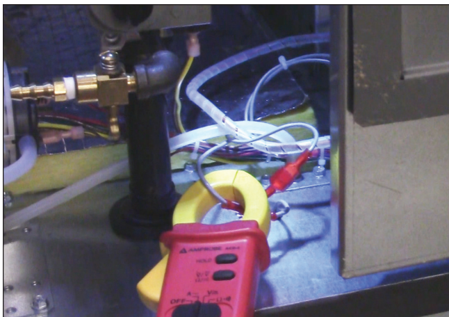
Figure 42. Amp Meter looped around an HSI wire.
