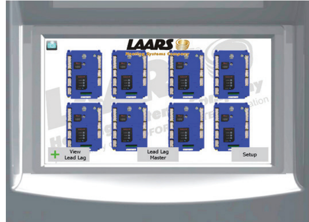
Figure 25. Touch Screen, shown with the ‘home’ screen of the lead boiler in a four boiler configuration, all conditions normal.
